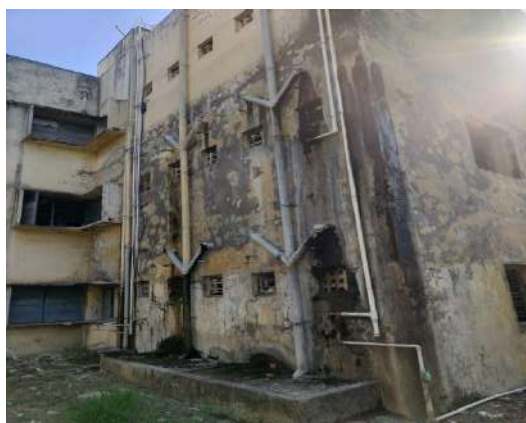
AFFECTED PIPE SYSTEM
