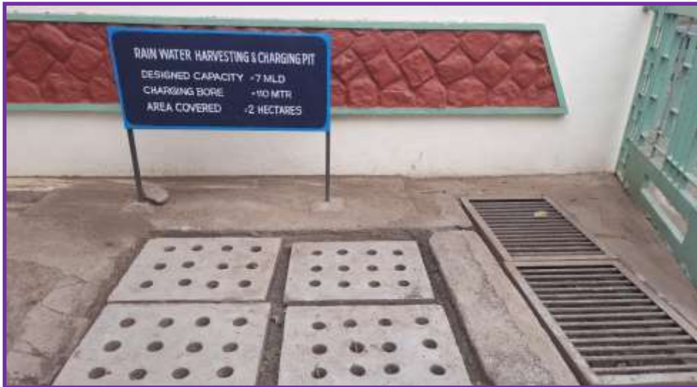
Sample Name Board in front a Rain Water Harvesting System
